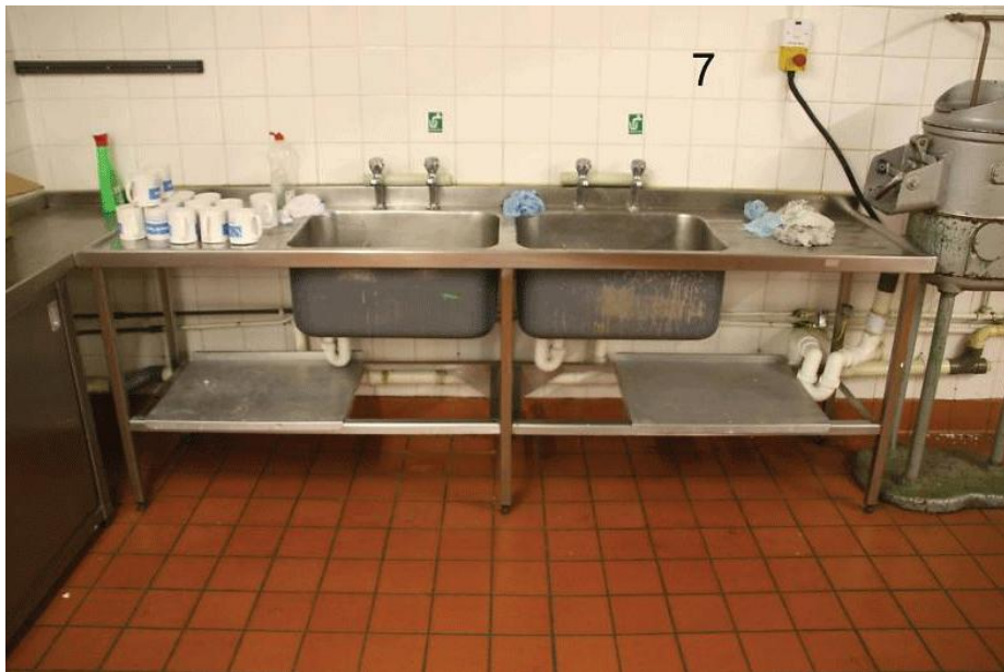
Stainless steel worktop with built in double sinks from a commercial kitchen. There is some paint on the front of the sink bowls. This unit is about 34" to 36" (875mm to 925mm) tall and has adjustable feet to help make the heights match where they are installed. Is is 23 5/8" deep x 94 1/2" wide (600 x 2400)
